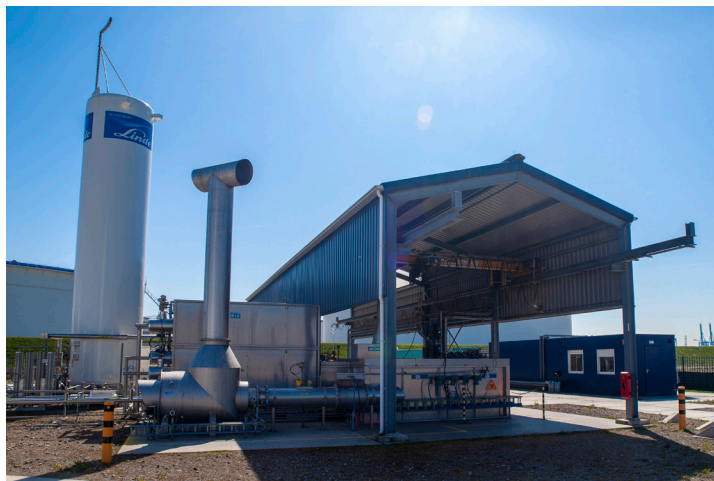
Figure 1. VSL's LNG mid scale loop calibration facility.
