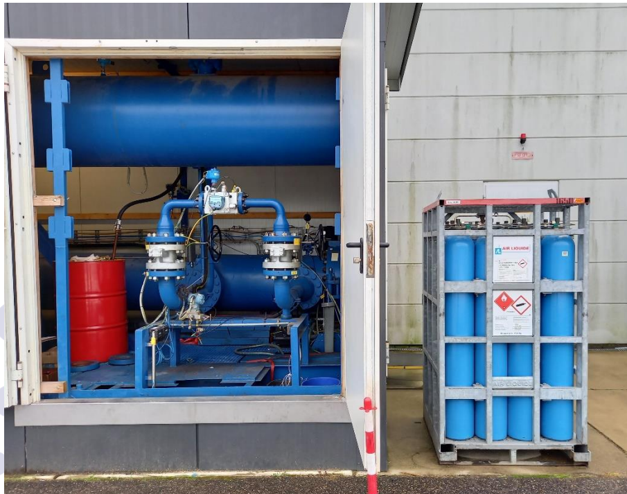
Figure 1. MuT mounted on VSL's GOPP, accompanied by hydrogen gas cylinders.
